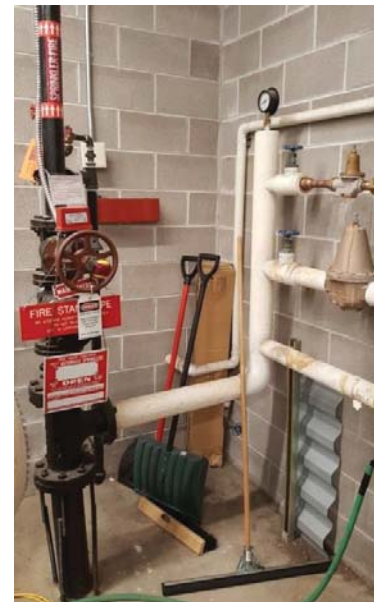
Figure 2 - Existing Fire/Water Main
