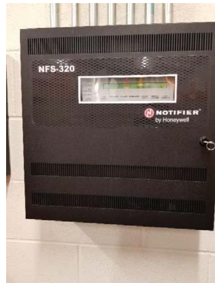
Figure 7 – Fire Alarm Panel
