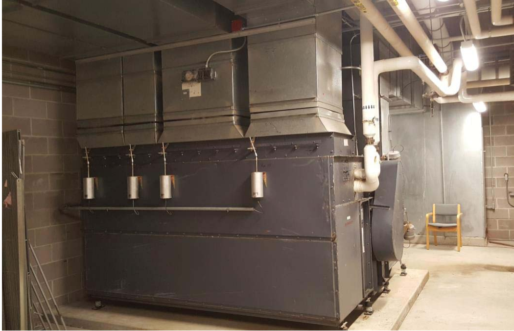
Figure 5 - 1981 Addition Multizone System
