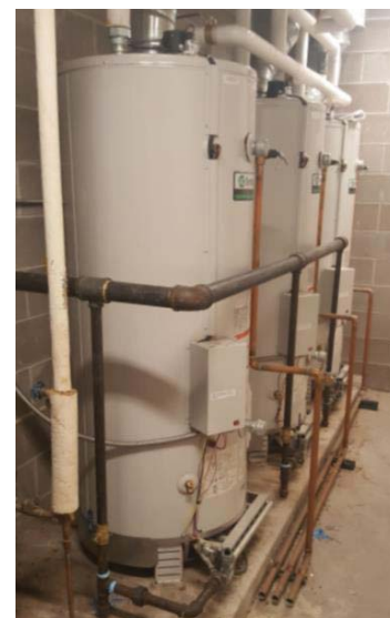
Figure 3 - 1981 Addition Water Heaters
