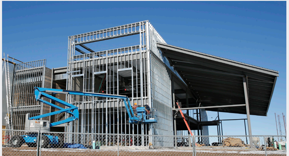
Work continues on the steel framework of the Flexible Industrial Technology Building. Michael Smith/LCCC
