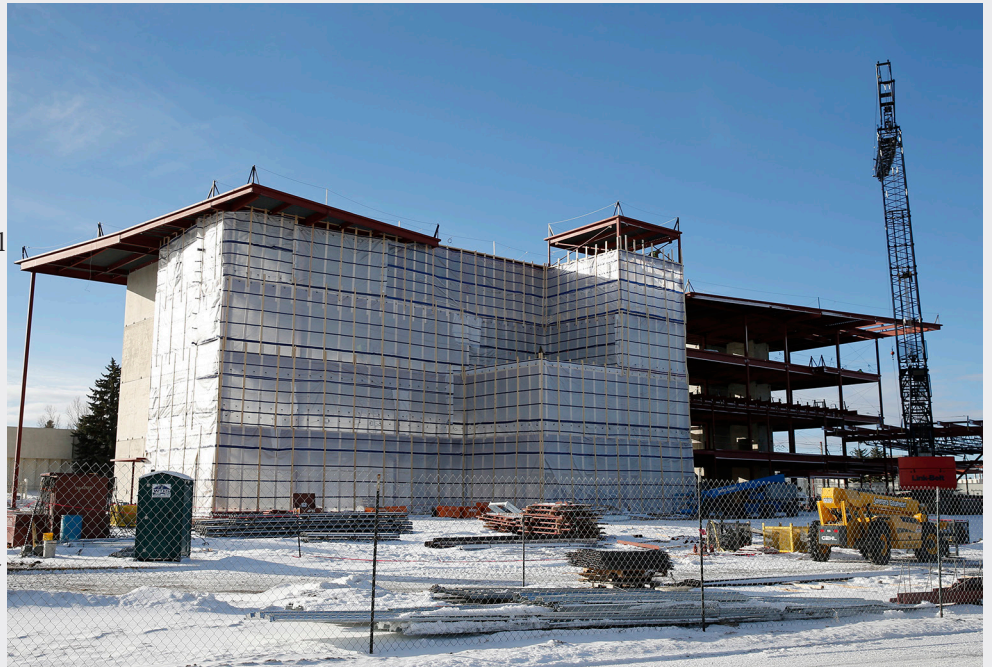
Plastic sheeting encloses the Student Services/University Center as crews work on interior structures. Michael Smith/LCCC
