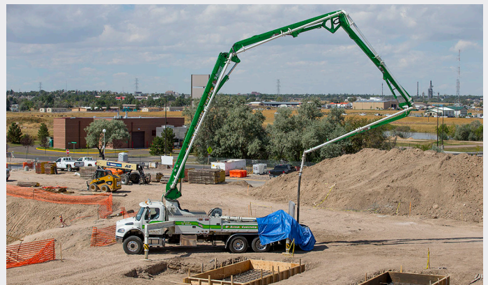
Crews make progress on the new Student Services & University Center. Ty Stockton/LCCC
