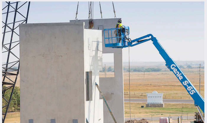
A close-up shot of the work on the walls at the Flexible Industrial Technology Building. Ty Stockton/LCCC
